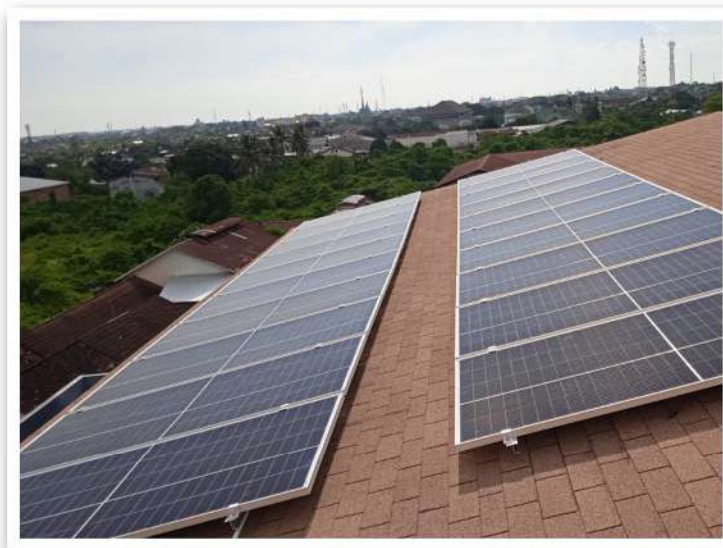
@ Lombok - 10 kW On Grid
