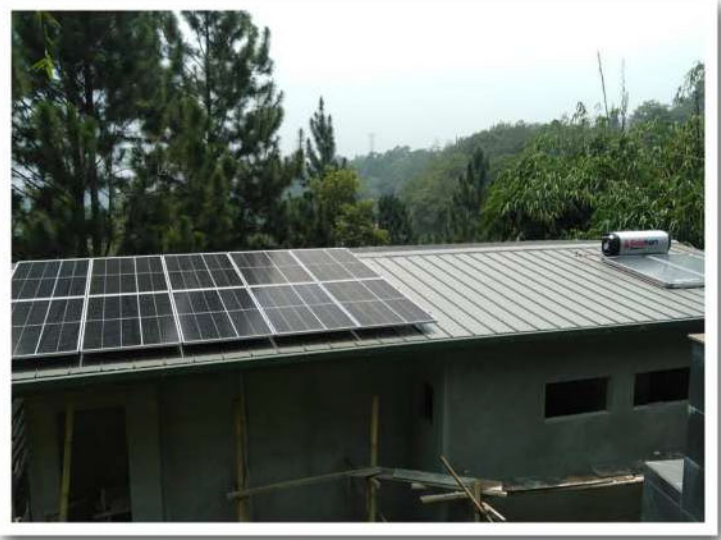
@ Bandung - 5 kW On Grid
