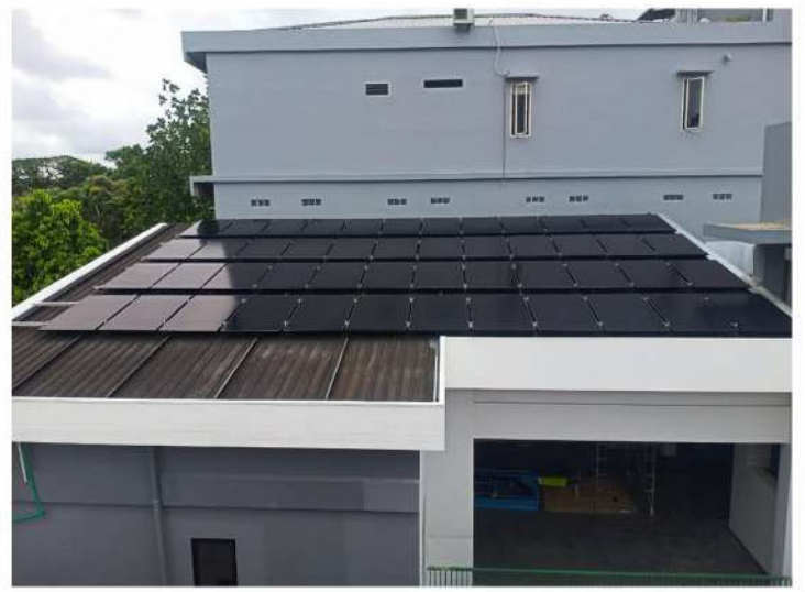
@ Ambon - 15 kW On Grid
